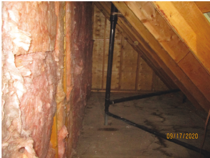
Photo 3: Shows west side attic space. Note 2"x8" rafters and 2"x6" insulated wall between upstairs bedroom and attic space.
