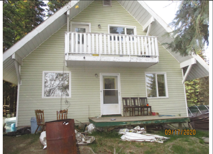
Photo 2: Shows east side of the house. Note balcony off the upstairs bedroom and main floor sundeck off the living room.
