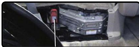
300V Hybrid Battery Manual Disconnect
