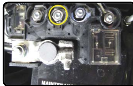
Main Fuse Box Power Supply Cable
