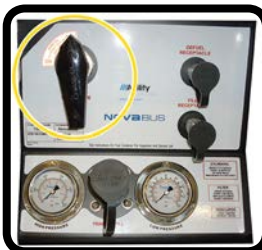
Emergency Shut-Off Valve (OFF position)
