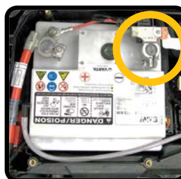
12V Battery Disconnect In Front
