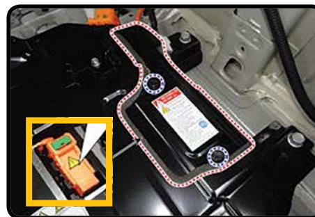
Service Disconnect Located in Trunk
