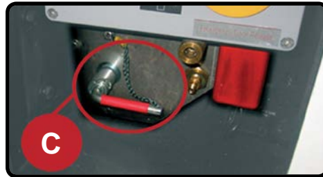
24V Battery Switch
