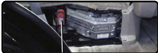
300V Hybrid Battery Manual Disconnect
