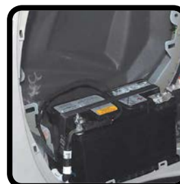
12V Battery Location
