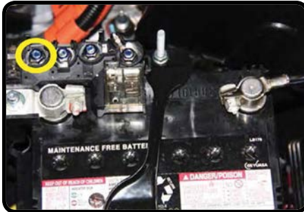
DC to DC Converter Connection
