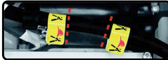
Cut 12V Battery Positive Cable As Marked
