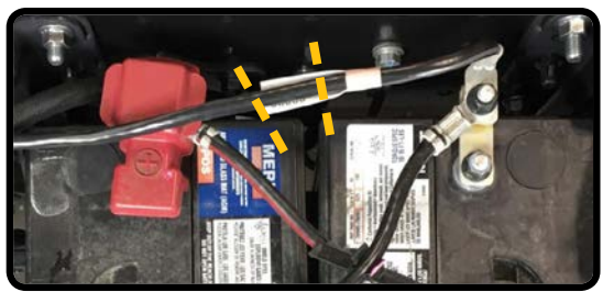
Cut Section Out of the Negative Cable
