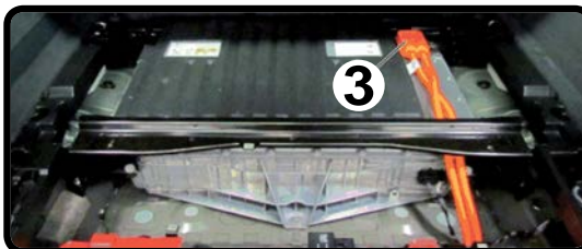
HV Disconnect in Trunk
