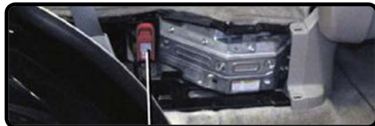
300V Hybrid Battery Manual Disconnect
