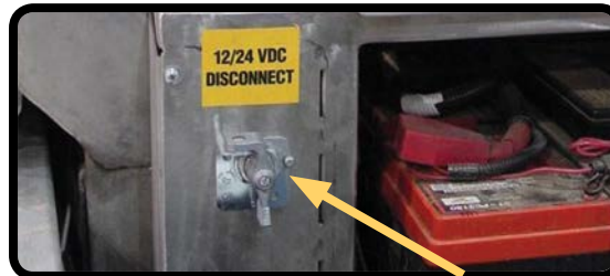
Emergency Disconnect (OFF position)
