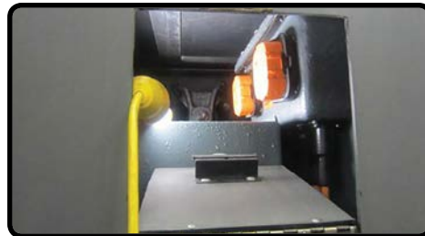
Access Door and MSD's
