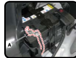
12V Battery In Trunk
